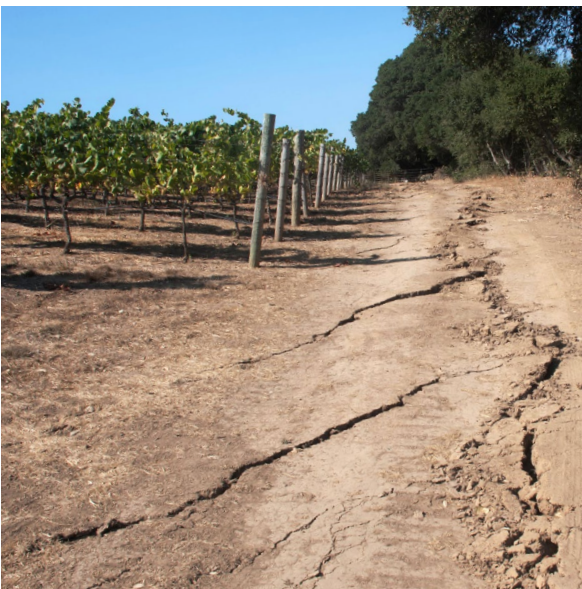
Surface fault rupture in Napa. Photo: CGS
