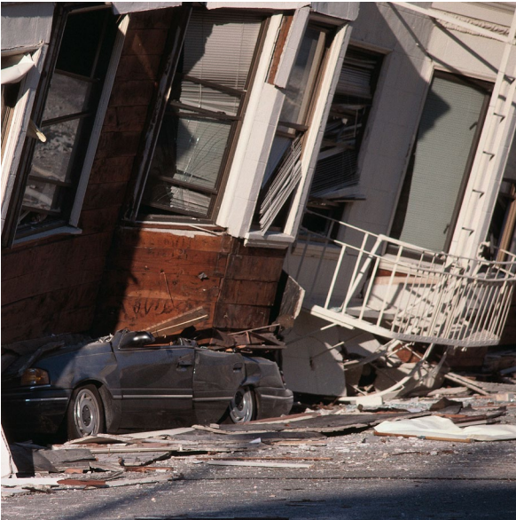
Liquefaction damage in the Marina District. Photo: USGS
