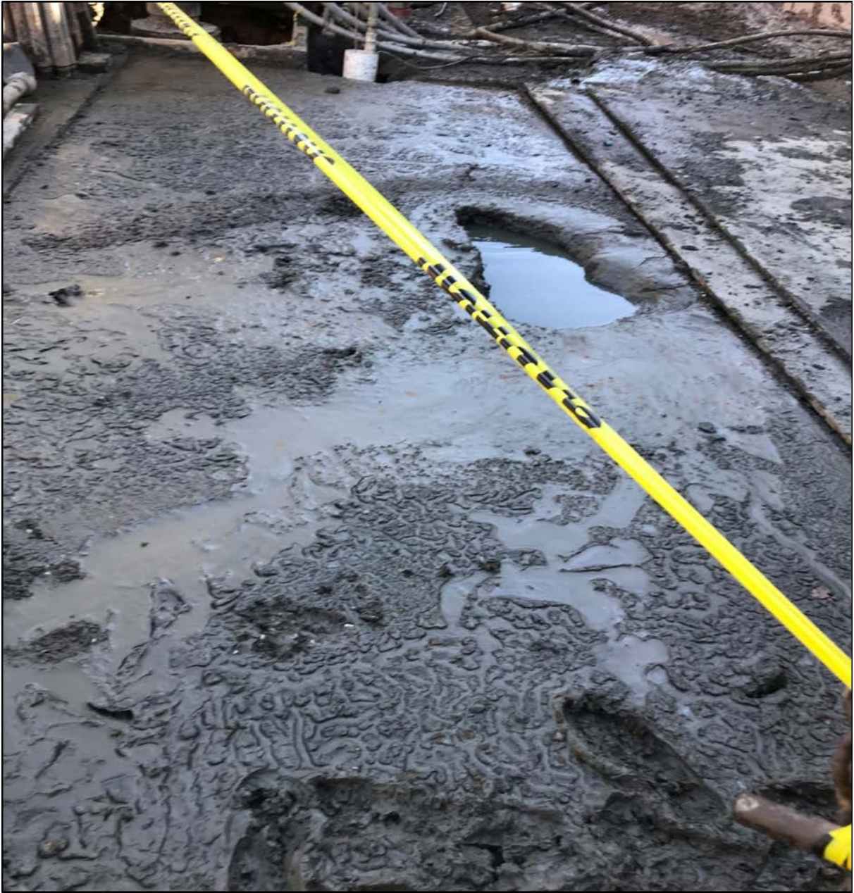
Figure 7. Photograph of drilling mud blowout and surface broach at Dow RGC 10 pad taken by InterAct on December 28, 2018.
