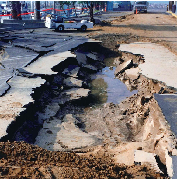
Liquefaction damage at Redondo Beach. Photo: CGS
