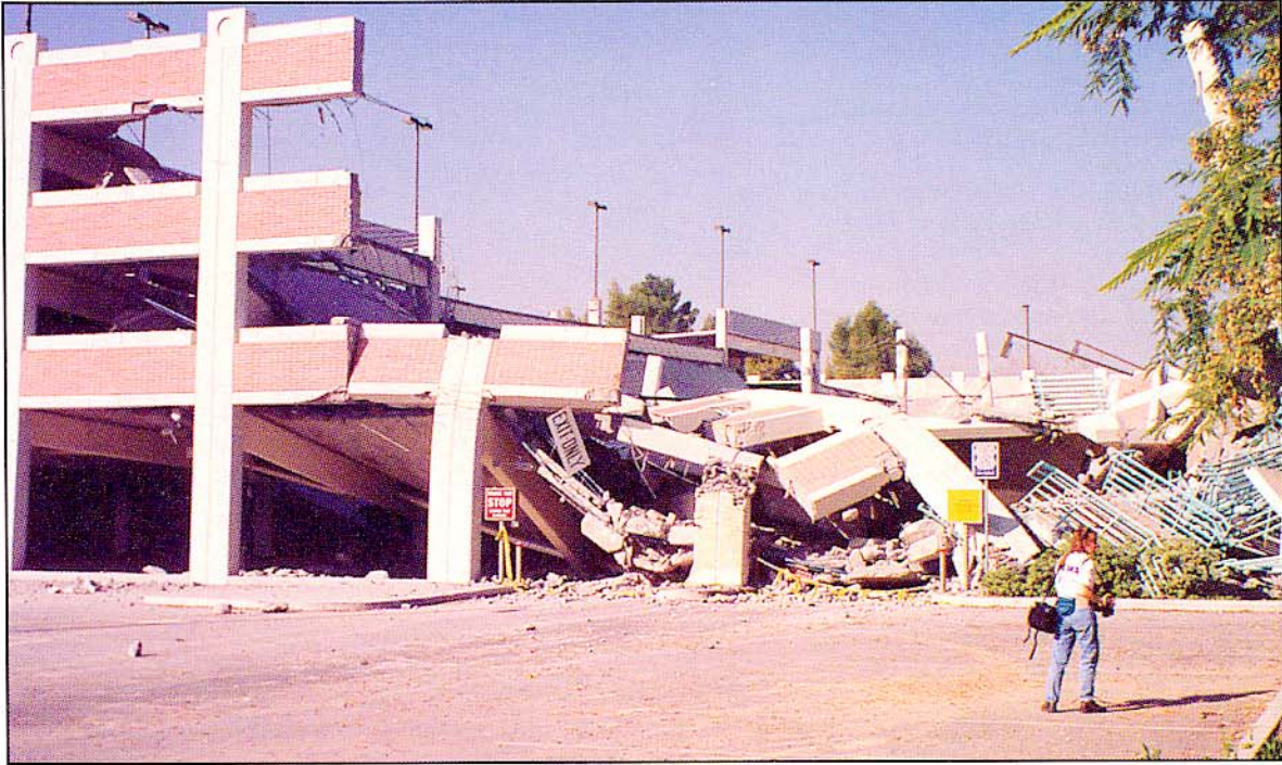
The California State University, Northridge parking garage after the January 17, 1994 Northridge earthquake. This is an example of violent shaking (see the Simplified Intensity Scale on page 167). Photo by Gerald R. Schimke.
