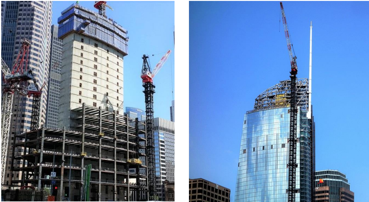
Figure 3. View of the concrete core wall and steel gravity system for Wilshire Grand Tower (left), and the rooftop sail structure and spire (right).
