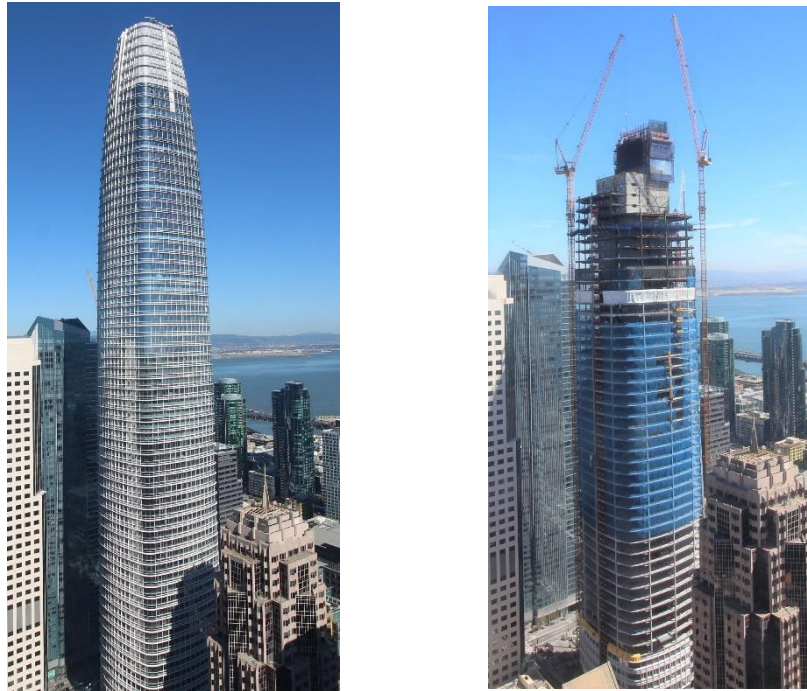
Figure 11. Views of Salesforce Tower after (left) and during (right) construction. The reduction of the concrete shear wall core at Level 50 can be seen in the right photo.
