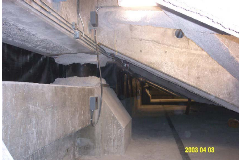
Figure 5. Sensors 7 (above isolator) and 2 (below isolator) with protecting boxes and cabling conduit installed on the east side of the basement at the Oakland City Hall to measure vertical motions.
