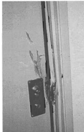
Figure 33. Doors had to be opened with sledge hammers (Naeim, 1997).
