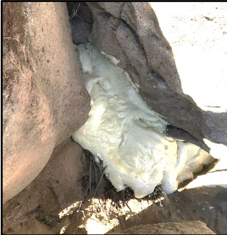
An AMLU contractor (bottom center of photograph above) examines a hazardous shaft on U.S. Bureau of Land Management (BLM) land in Kern County that was discovered near multiple residences by a homeowner's young son. The mine shaft was subsequently sealed with expanding polyurethane foam (PUF) (left). The PUF plugs were then covered with soil, leaving no sign of the shaft. Photos: DOC (2018)
