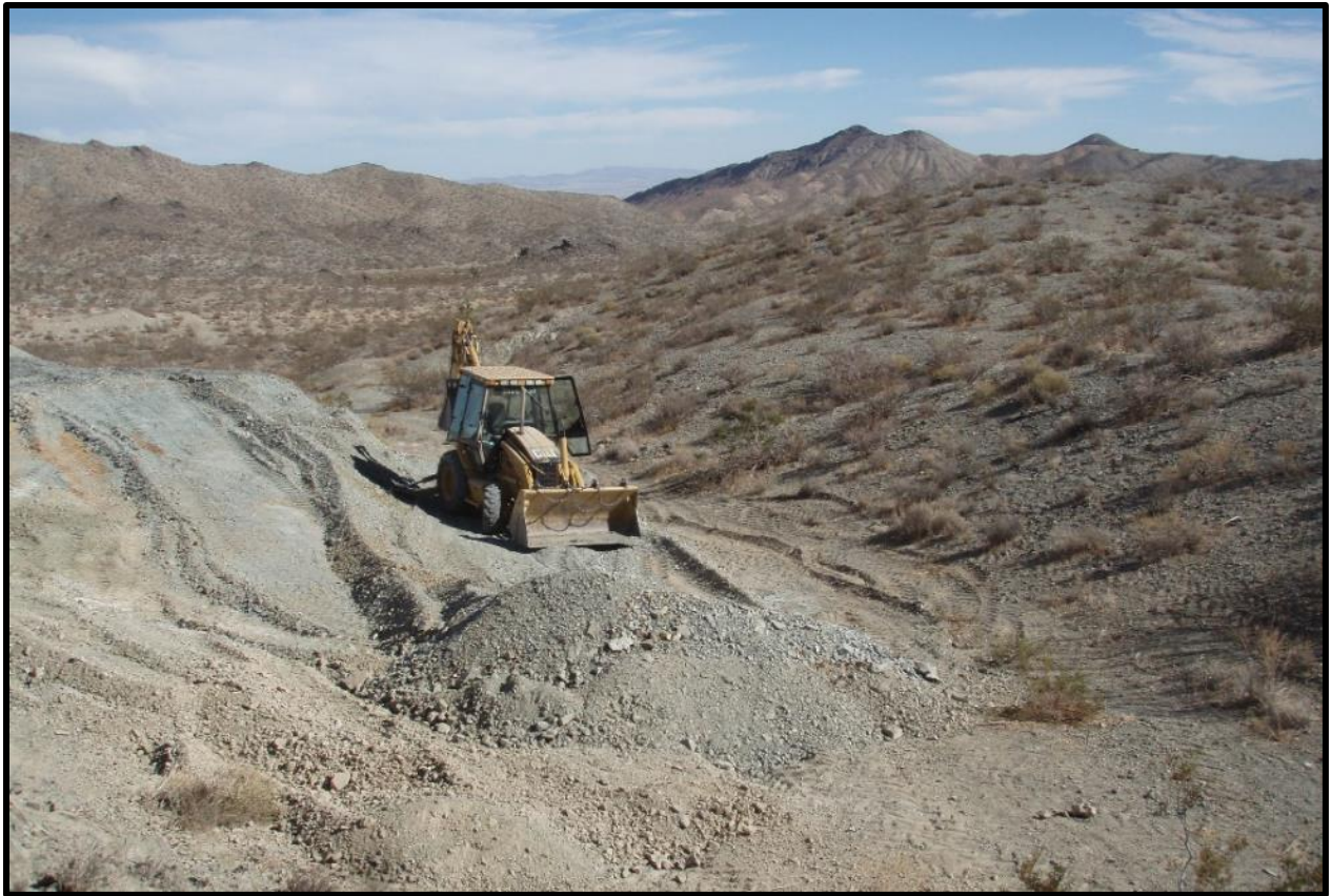
Fencing installed around a hazardous mine shaft adjacent to a dirt road on State land in San Bernardino County. An AMLU contractor later permanently backfilled the opening, which was increasing in size, with a backhoe using onsite material. Photos, DOC (2002-2007)
